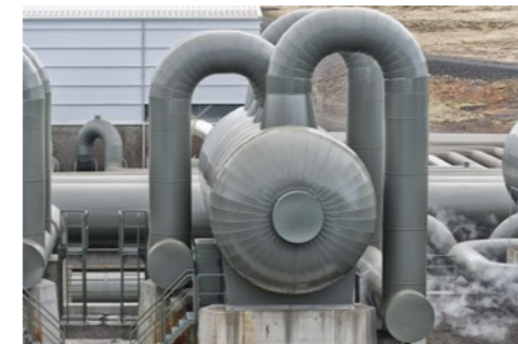
• the water supply pump station
